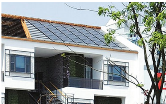
Fig. 3.25 Solar energy system on south sloped roof
